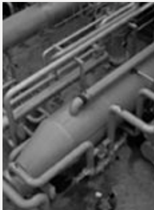
Pipelines & Pumping Stations
