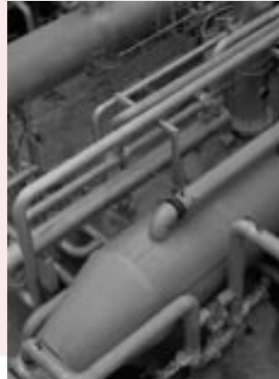
Pipelines & Pumping Stations
